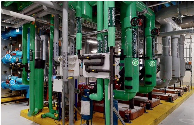
FIG. 4 — MECHANICAL SYSTEMS CAPTURED WITH OVERHEAD PIPING AND LABELS INTACT.
